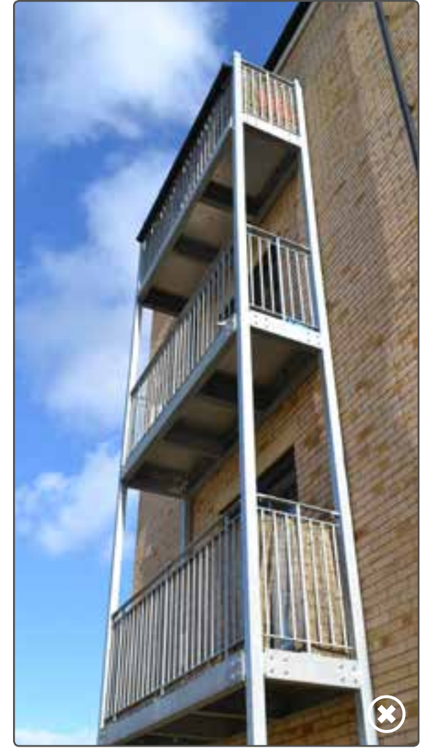
Poor external balcony design
