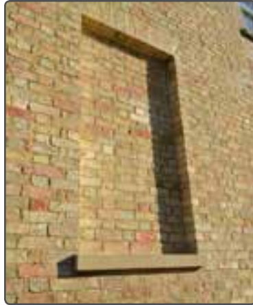
A simple bricked in dummy window with a reveal can add relief to a wall - Huntingdon
