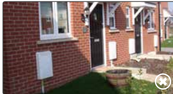
Poorly located meter boxes - St Ives
