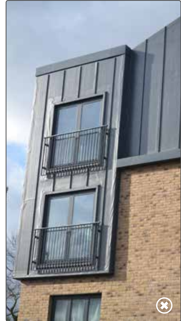
Here we can see this applied material bubbling up
