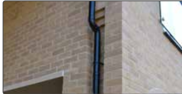
Carefully disguised pipework - Huntingdon
