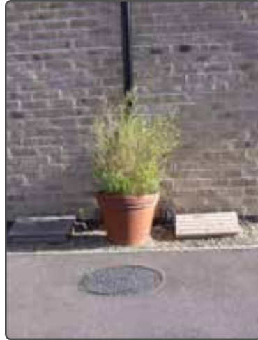
Semi concealed gas meter
